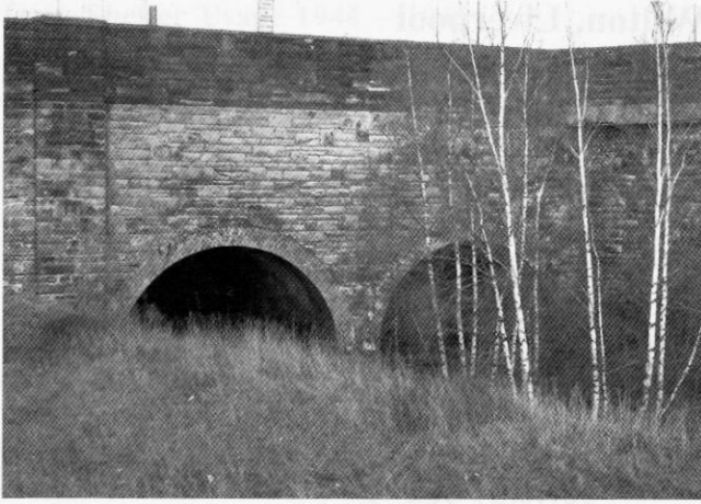
The southwestern portals of Walton-on-the-Hill No 3 Tunnel in February 2005 taken from the nearby Kirkdale Station. Only the tunnel on the left ever saw trains. The tunnel on the right runs parallel for almost its entire length but finishes at a dead end just before the Selwyn Street cutting. Photo by Paul Wright
